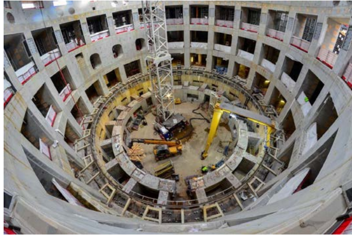
800 tons of concrete and over 200 tons of steel are being used for the Tokamak building.
